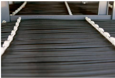
Water evaporates as it travels through the cooling towers
